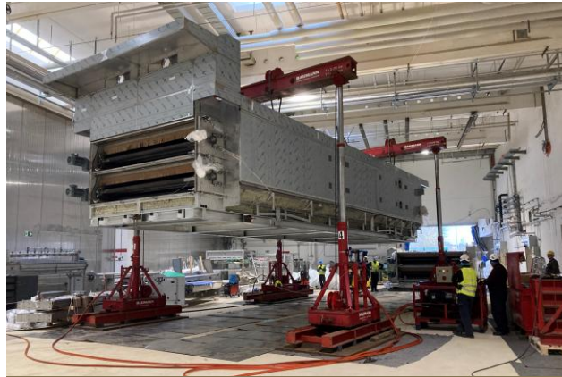
State-of-the-art stone oven in Eisleben, Germany, for new artisanal bread line
