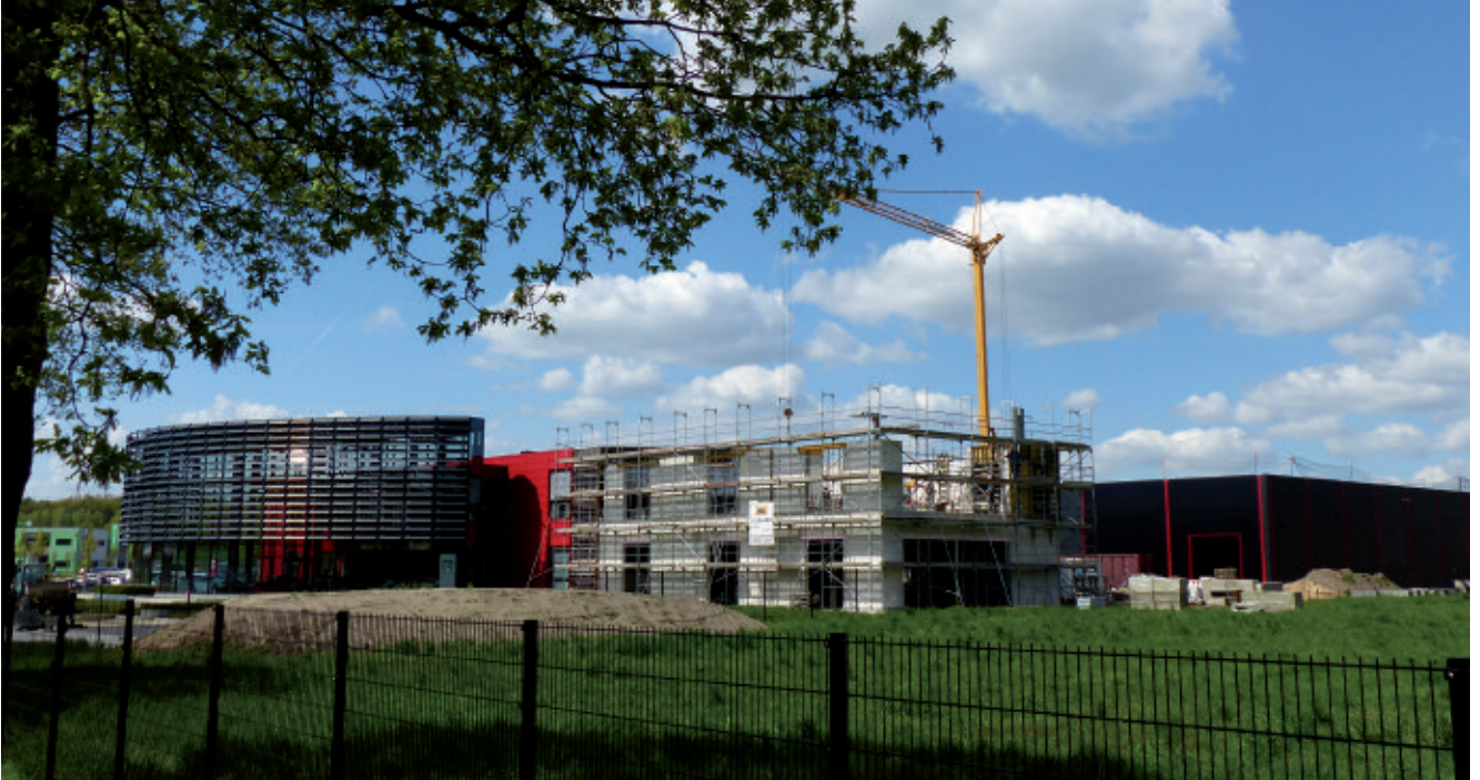
Extension of the office building in Artegastraße in the summer of 2016 (Development Voltabox and Body Kinematics)
