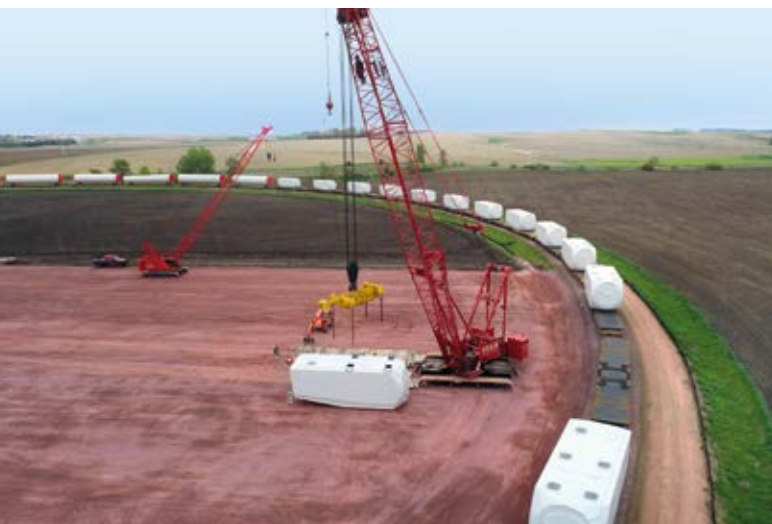
Transportation of nacelles and tower segments by rail to the construction site
