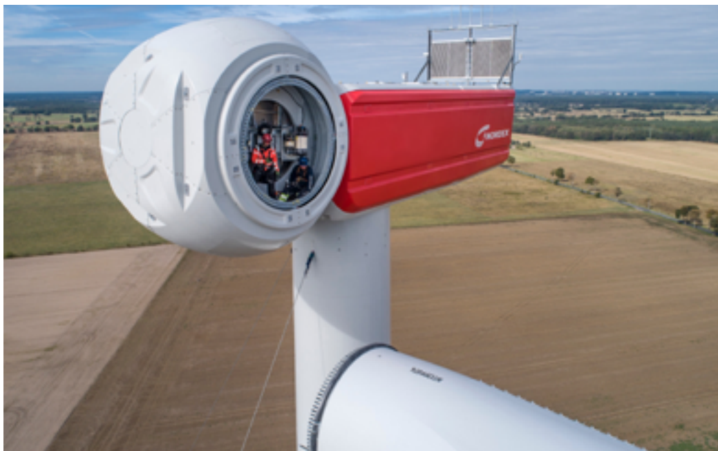
Ensuring sustainability through highly efficient energy generation: Employees assembling a Delta4000 N149/5.X in Genshagener Heide, Germany
