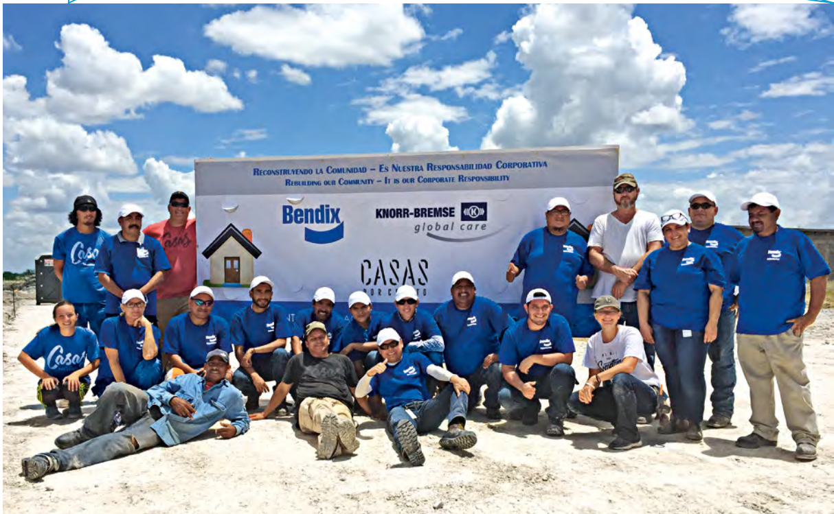
Knorr-Bremse employees built the first of 20 houses for tornado victims in Acuña, Mexico.
