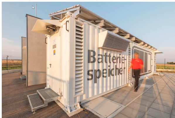
Utility-scale battery storage
