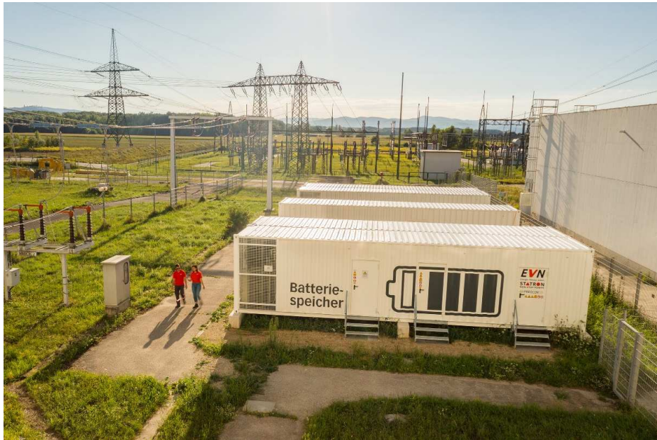
5 MW battery storage pilot plant in Theiss
