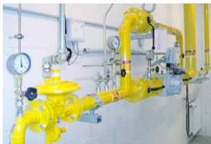
Natural Gas (LNG)
